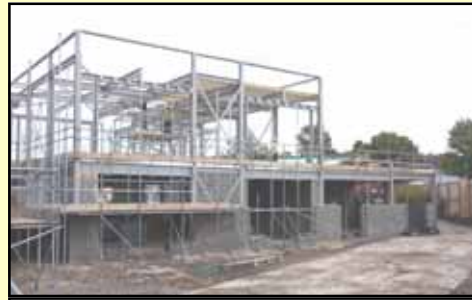
Community Area - Steel Frame in Place. Roof, Brick and Blockwork in progress.
